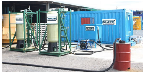
NORM Filtration System
