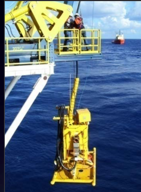
Installation and Workover Control Systems
