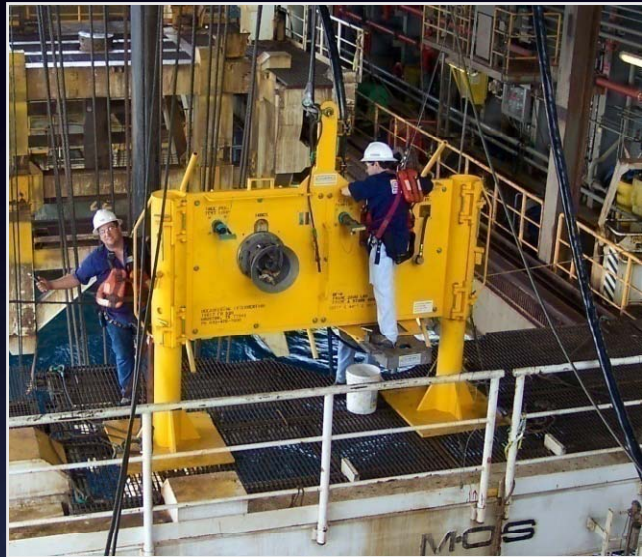
Installation Workover & Control Systems
