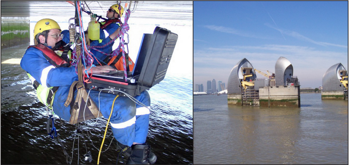
Oceaneering Rope Access technicians carrying out TOFD survey of the Thames Barrier, London.
